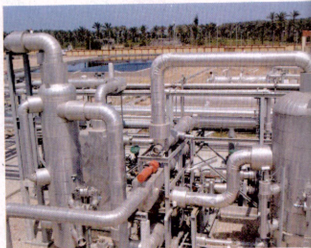
Dana Gas Egypt's El Wastani gas-processing facilities in the Nile Delta. www.danagas.com
